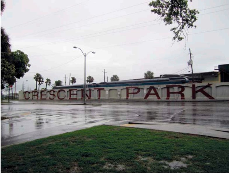
Abb. 4: Crescent Park Flutmauer, in der Nähe des French Market, New Orleans, April 2013 • Foto: Alice Mah
